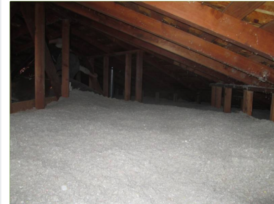
Cellulose attic insulation
